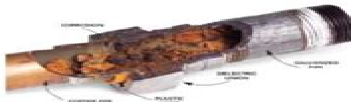
Fig 1: Corrosion in Pipelines
