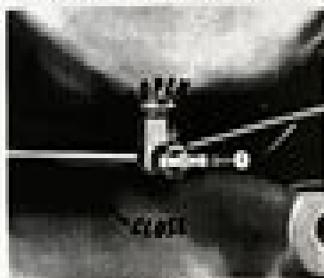
Figure 6 Fuel Shut-Off Valve
