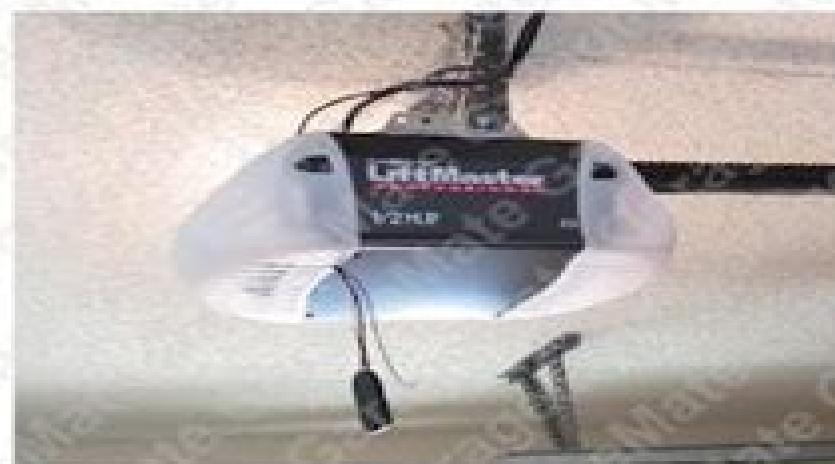
Garage Mate Receiver Installed
