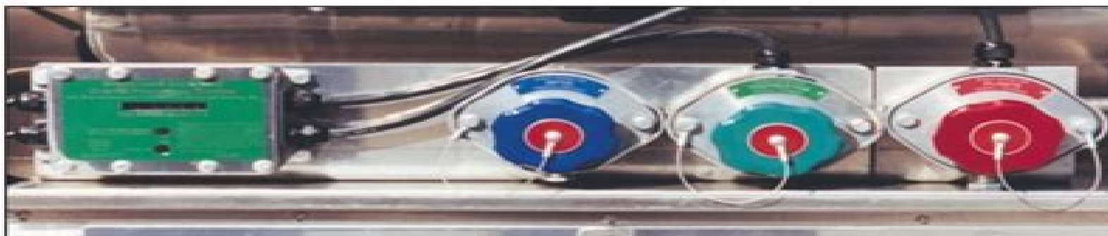
Scully truck mounted control monitor and sockets
