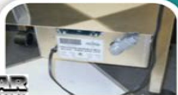
Pump Mounts Under Distiller's Storage Tank
